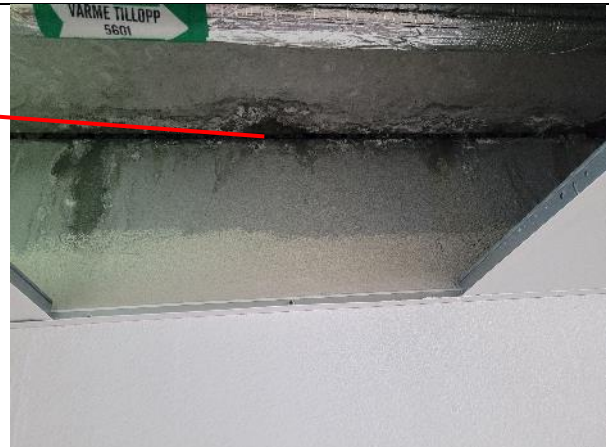
Fuktskador ovan undertak
